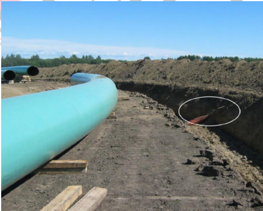
Excavation may unearth wires
