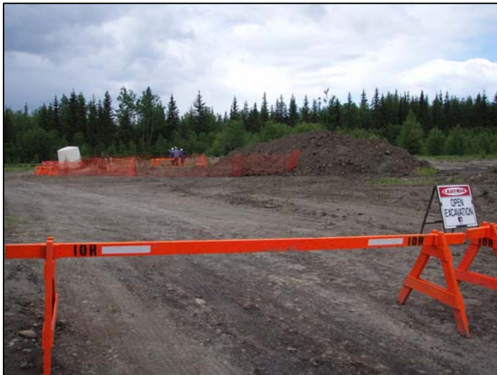
Properly secured site with lease entrance barricades and fully erected snow fence
